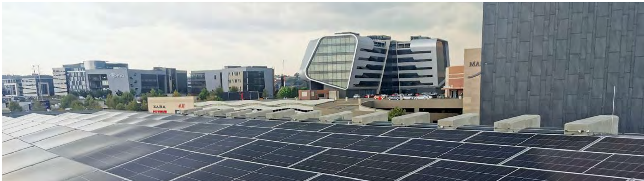
Rooftop PV system at Nexus Waterfall, building 1 with Gateway West and The Ingress in the background
