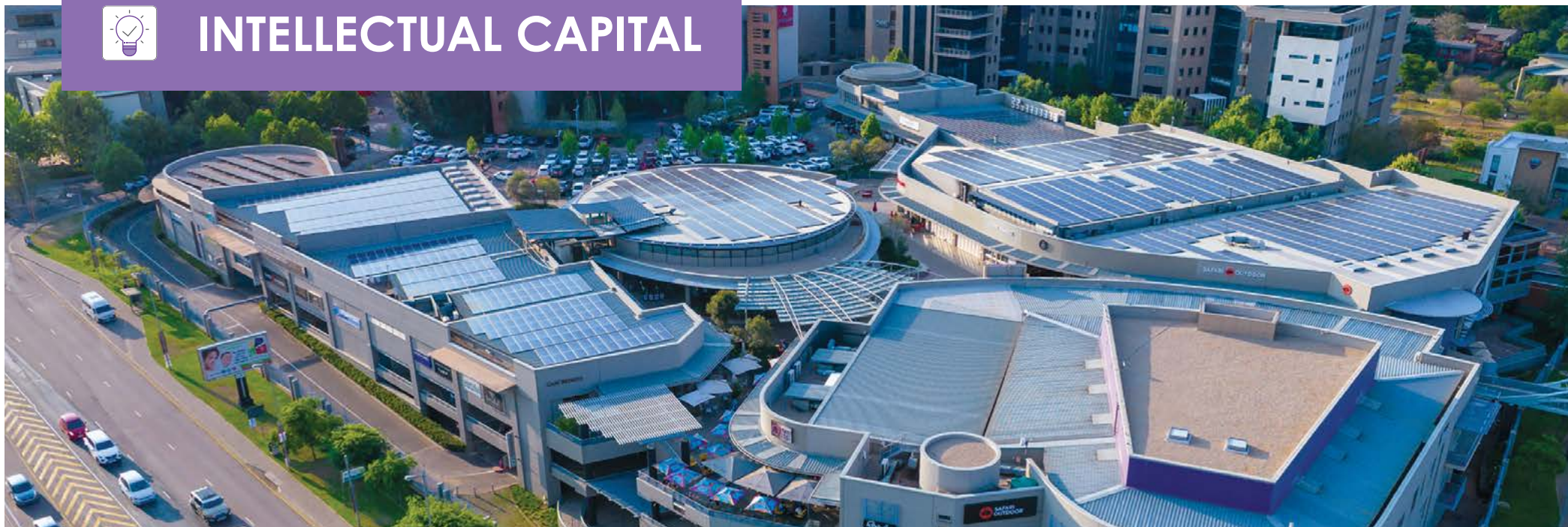
Rooftop PV systems at Lynnwood Bridge - Retail, City of Tshwane
