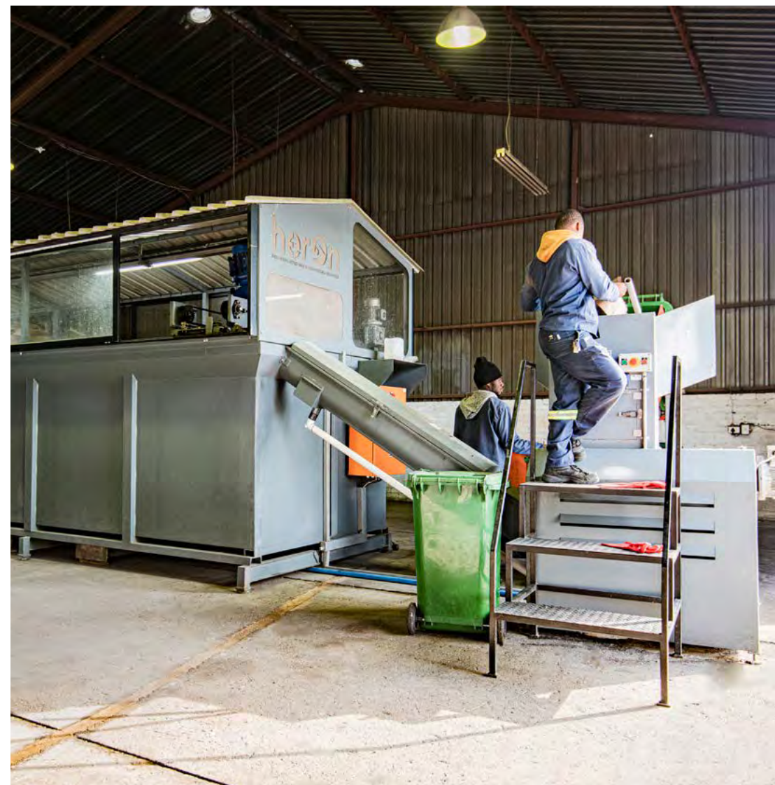
Our onsite in-vessel composter machine (Heron IVC), processing wet waste generated in Waterfall City, reducing waste to landfill
