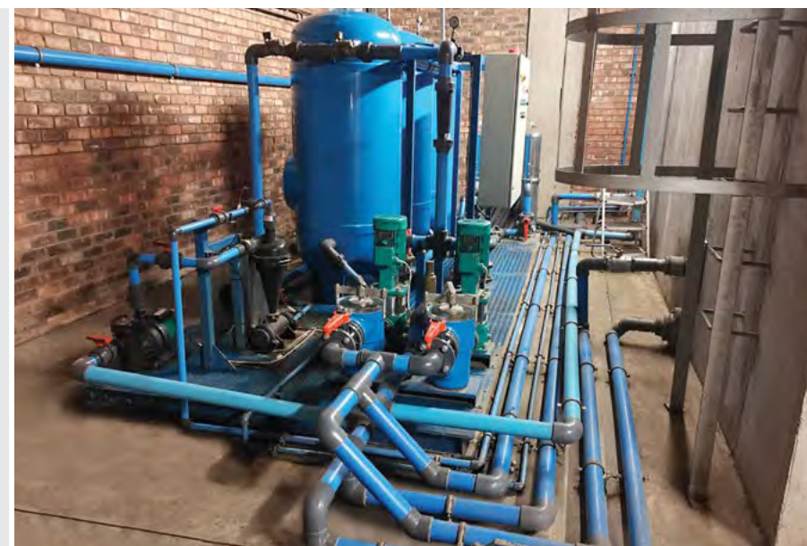
Grey water filtration system in the basement of Mall of Africa, Waterfall City
